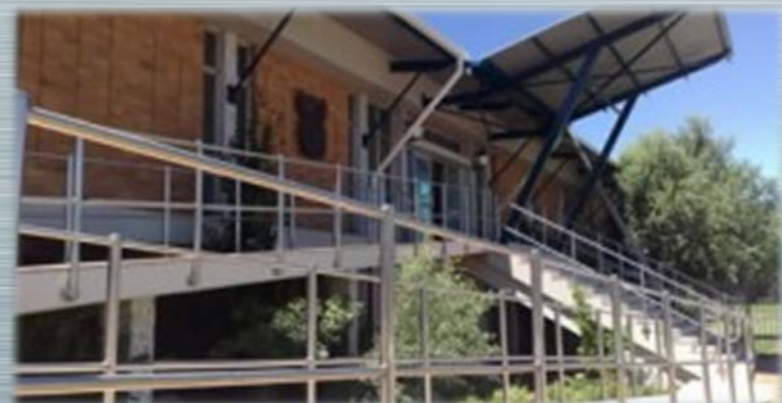
MVD Kalahari was appointed as Structural Engineers on the R14m project to repair and renovate the Kimberley High Court.
